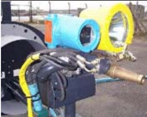
Front view of Cannon in manway with camera and lighting
