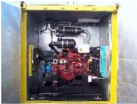
Acoustic Power House
