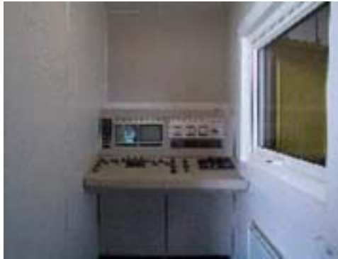
Acoustic Operator Control Room
